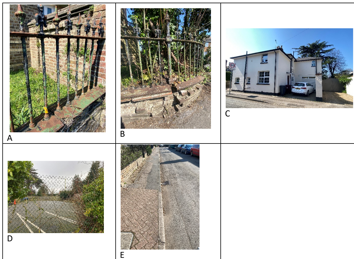
Figure 26 Images of loss or deterioration of details (Images Claire Truman)
