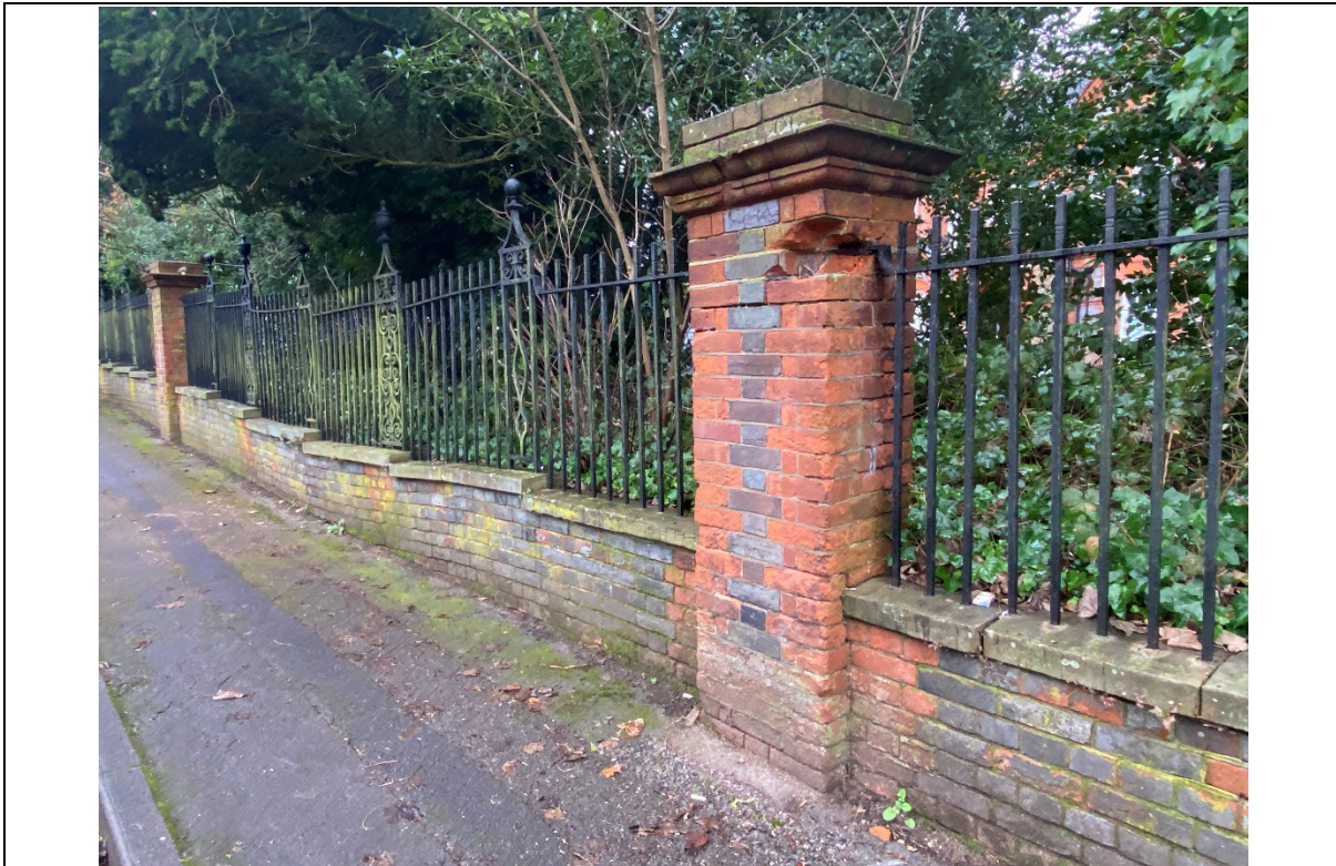
Figure 22 The brick piers and railings to Hillside are falling into disrepair – view along Lower Mount (Image Claire Truman)
